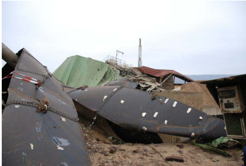
biogas plant in Riedlingen
